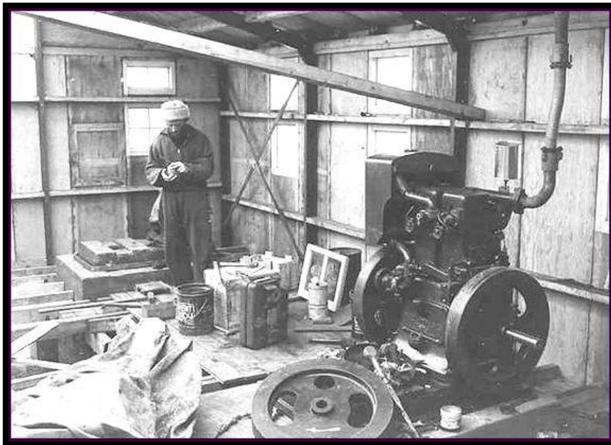
The new Generator shed nearing completion, with one of the Lister units in the foreground.
